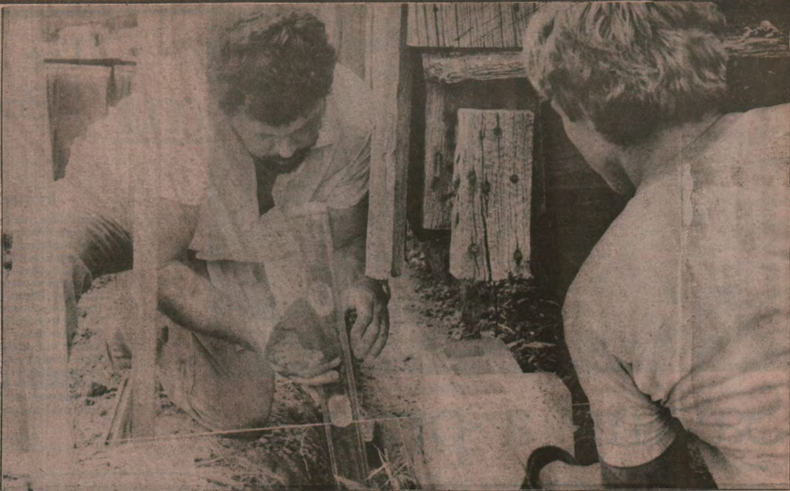
Don Murphy, Robinson, (left) and his son Garland (Bub) (at right) make the finishing touches on laying a corner block of the restaurant foundation. Murphy and his two sons (Scott is not pictured) took time out from their own masonry business to donate their skills and lay a new foundation for the old building.
