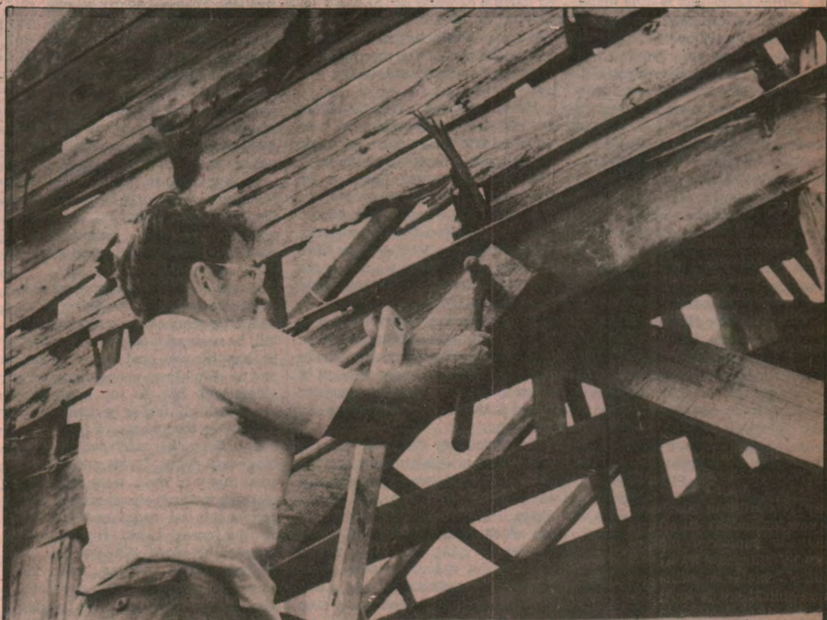
Journalism/history teacher Dwight Connelly, Martinsville, secures a wood brace on the side of the restaurant building.
